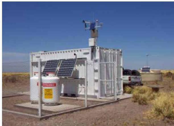
FIG. 2.11 – Le Central Laser Facility.
