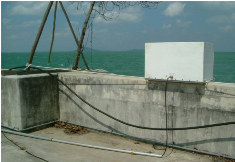
Figure 3.36: Final prototype with screened cables tested near sea in coastal configuration
