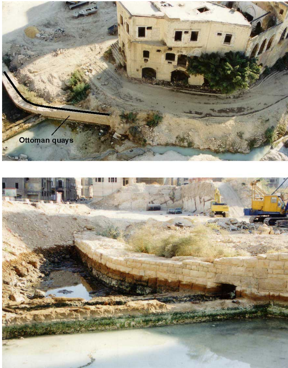
Figure 5.24: Ottoman quays unearthed during the EDRAFOR construction works (photographs courtesy of EDRAFOR). These quays lie just outside the ancient basin and attest to a gradual dislocation of the harbour coastline since the Bronze Age.
