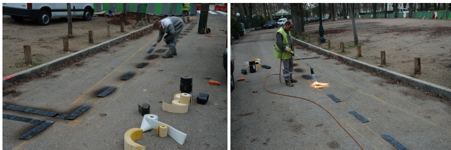
Figure 2.1: The road worker lays out pre-manufactured shapes in the design required. Once in place, a blow torch is used to melt the plastic on the surface of the road.
