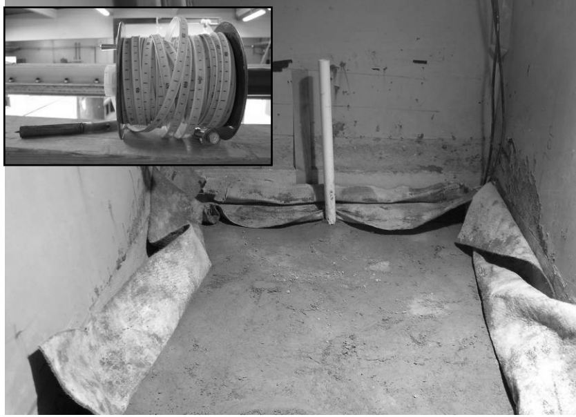
Figure 3.6 Water level observation well and indicator.
