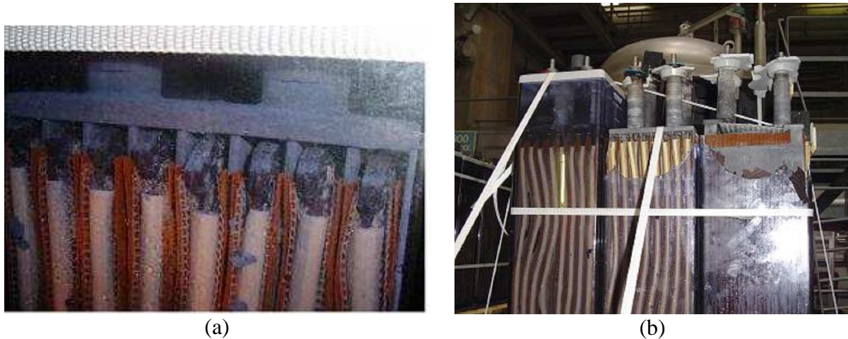
Figure 88: Due to corrosion, short-circuit took place and caused explosion accident in a standby tubular battery: (a) positive plate lengths were increased and touched the negative collective bar, (b) positive plates were distorted; the positive terminal obviously became more higher than the negative terminal; battery was destroyed after explosion (source: EDF).
