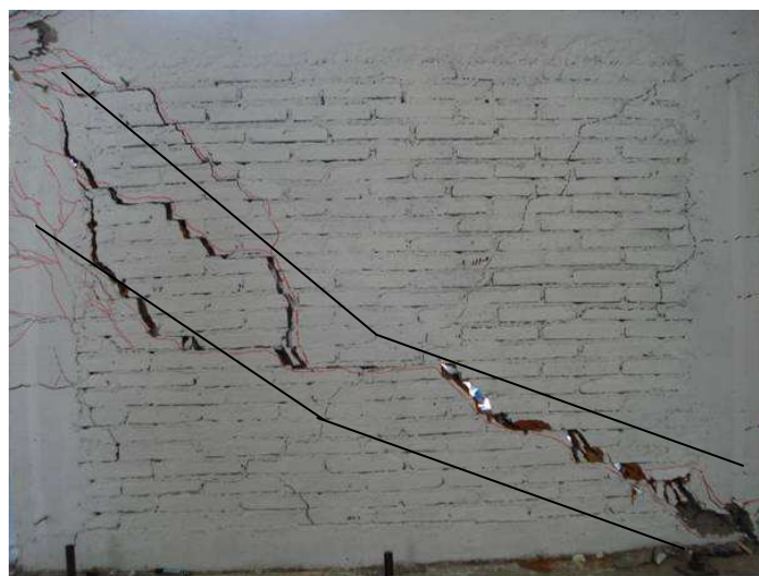
Figure 5.21: Final failure pattern for the wall MUR2
