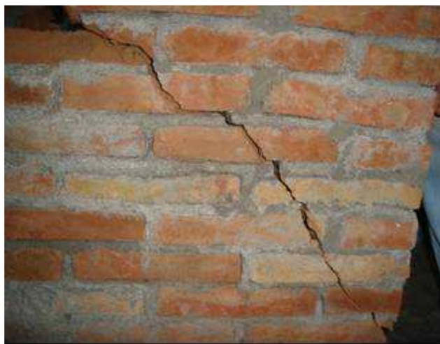
Figure 2.5: Masonry panel failure caused by units cracking and joint sliding
