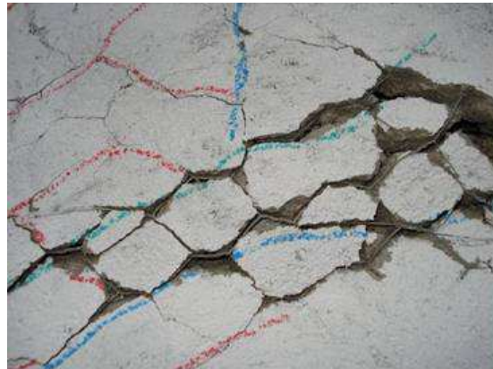
Figure 4.37: Final damage state of reinforcement at the upper corners
