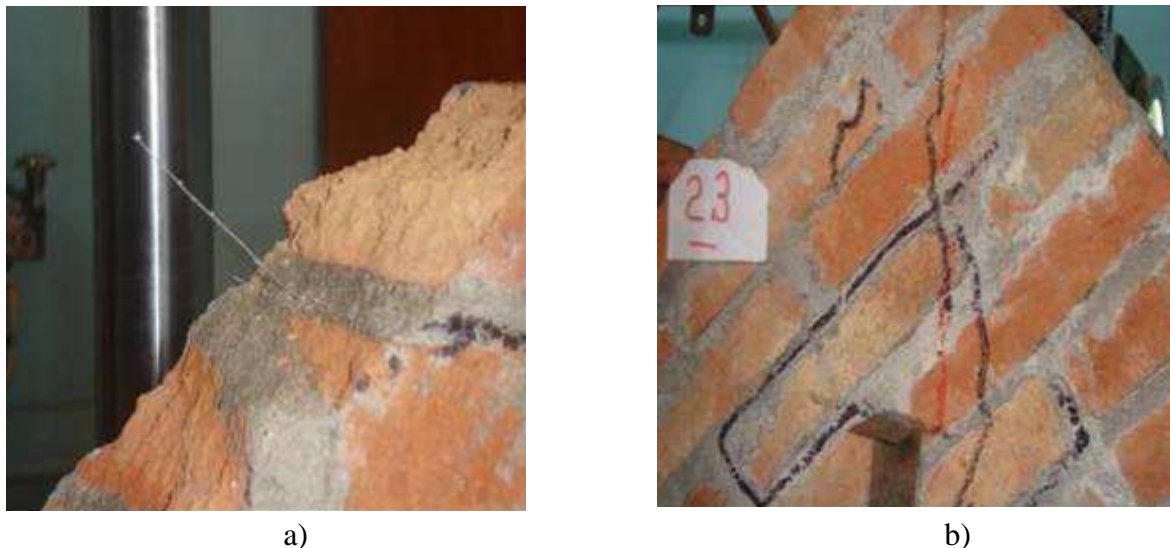
Figure 4.13: a) Tension failure of metallic reinforcement mesh in panel MR18, b) Failure mode of the panel MR23
