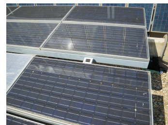
Pergola 5 array solar irradiance and temperature sensor
