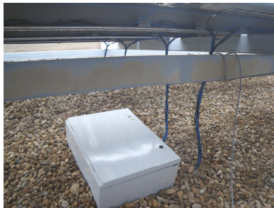
Closed connection box
