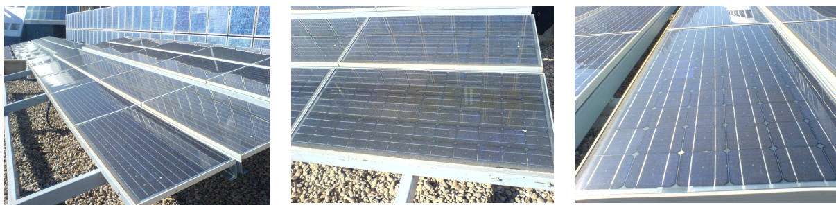
Pergola 5 array on clear day
