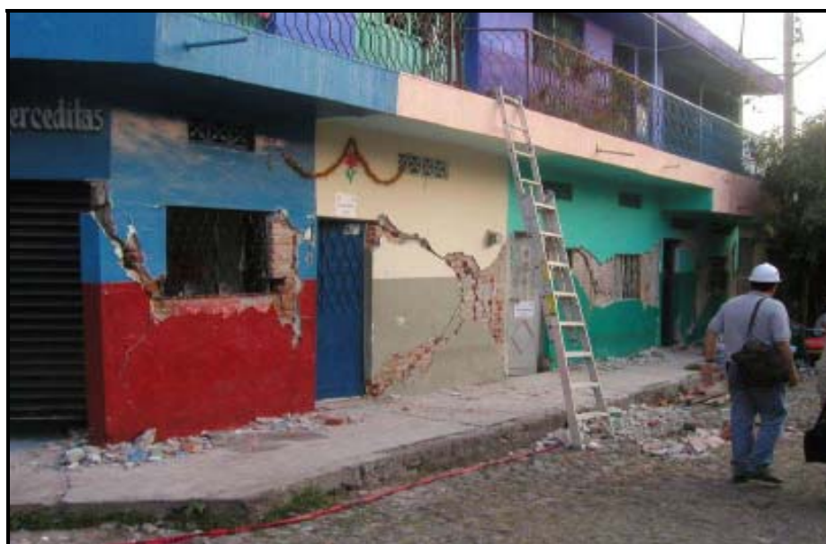
Figure 5 Common damage in the non-reinforced masonry [31]
