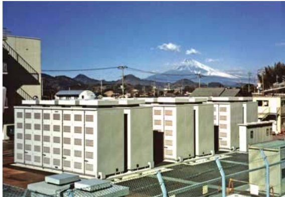
Figure I.4 NaS battery installation at Tokyo Electric Power Co.'s Ohito (6MW/48 MWh) [www.powermag.com]
