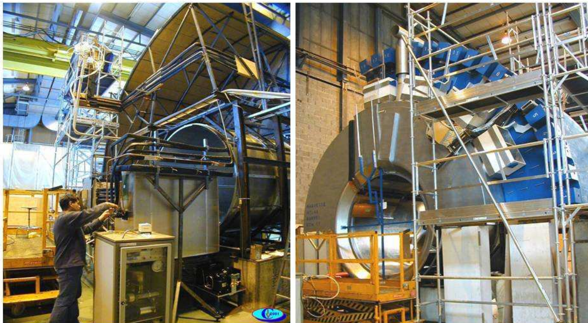
Fig. 4.23. 6kW evaporative cooling demonstrator and service model: arrival at the cold box of insulated coolant delivery and exhaust tube bundles from the flow and exhaust regulator racks (CERN Building 175).
