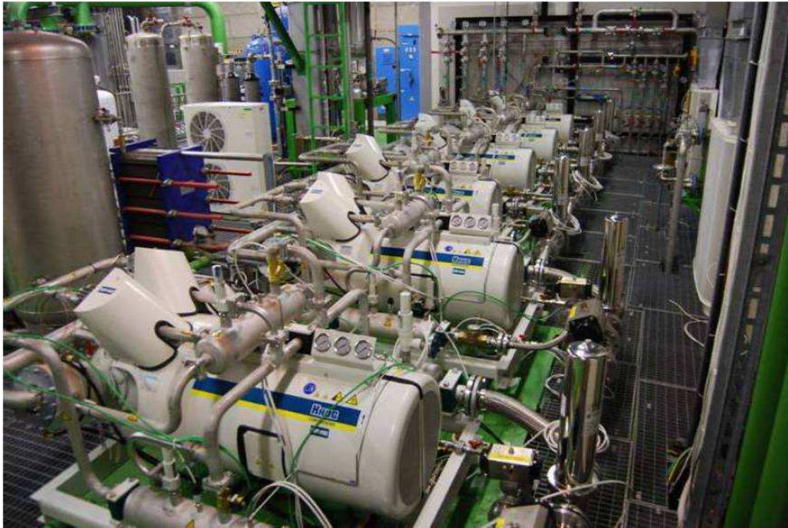
Fig.4.40. Compressor installation in ATLAS USA15 technical cavern for the C_3F_8 evaporative cooling system.
