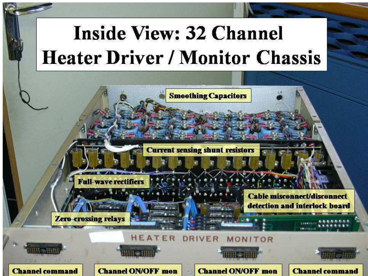
Fig. 4.32. Compact implementation (32 channels in 6U 19” chassis) of zero-crossing AC powered heater driver.
