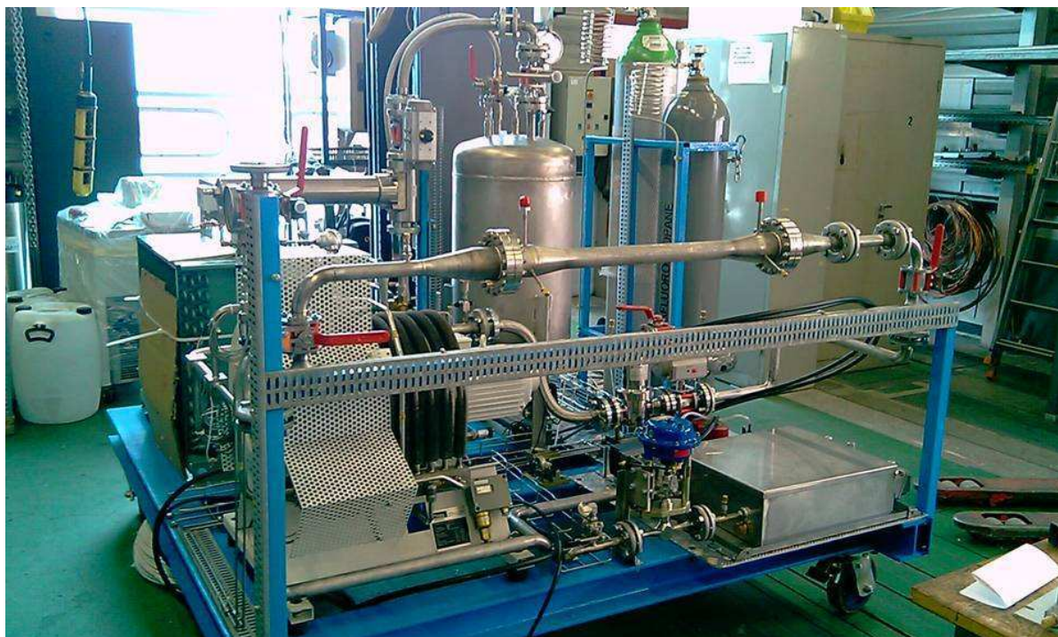
Fig.5.8 The ultrasonic flowmeter in a trial installation in the dedicated C_2F_6/C_3F_8 blend recirculator.
