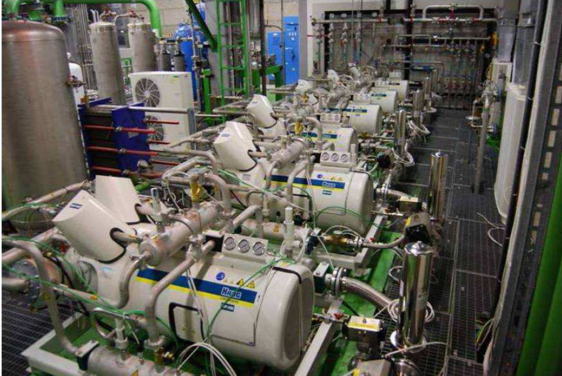
Fig.4.40. Compressor installation in ATLAS USA15 technical cavern for the C_3F_8 evaporative cooling system.
