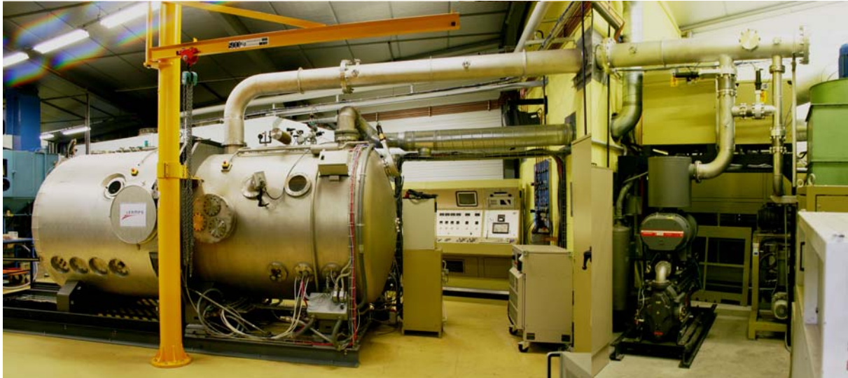
Figure II.11 Installation VLPPS après modifications
