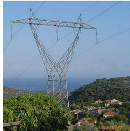
Fig. 3-10 : III insulator strings
