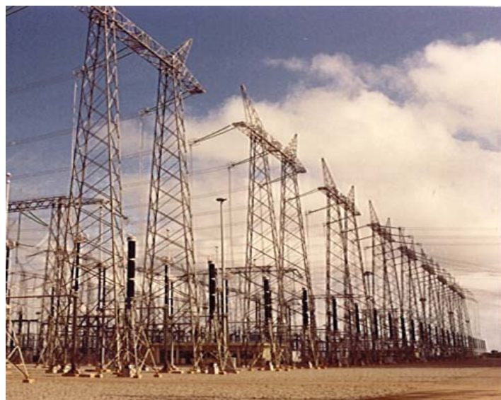
Fig. 3-44 : Gantries in substation
