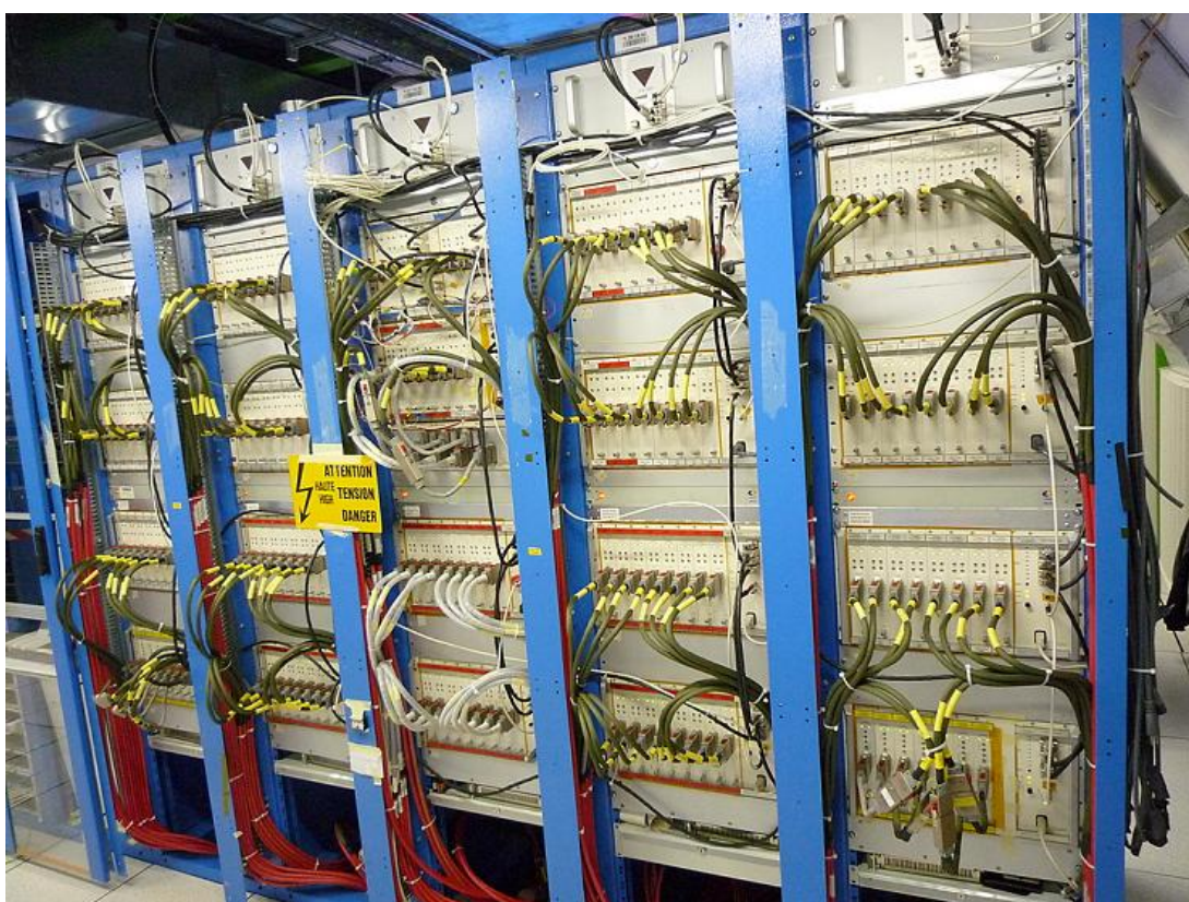
Figure 3.10: High-voltage power supply crates in USA15.
