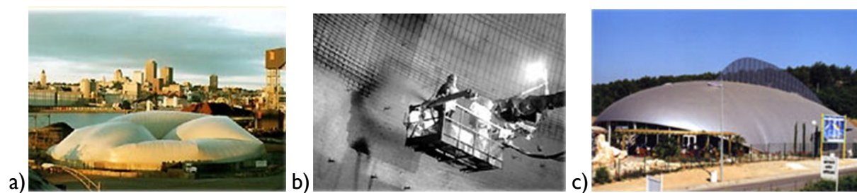
Fig. 2.51: a) Inflation of formwork; b) shotcreteing on the inside of the membrane; c) irregular shape structure constructed with pneumatic formwork [Pirs SA.]
