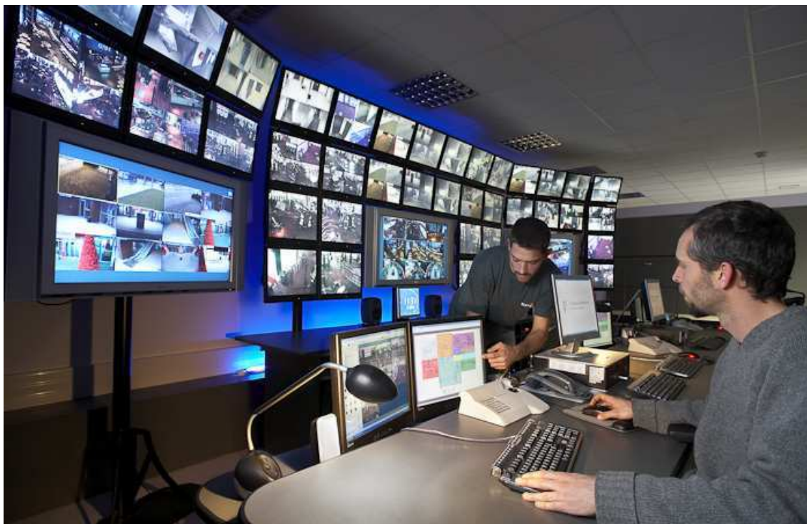
Figure 1.2 – A control room for video surveillance (source [securite-surveillance.com, 2009])
