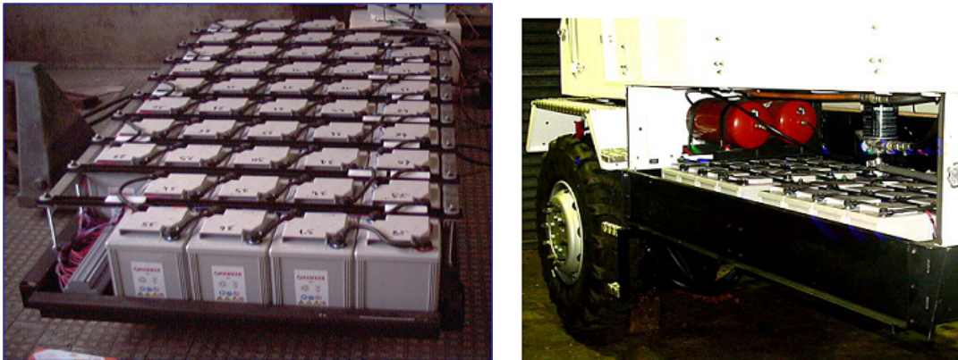
Figure 2.2: Lead-acid batteries implemented in ECCE
