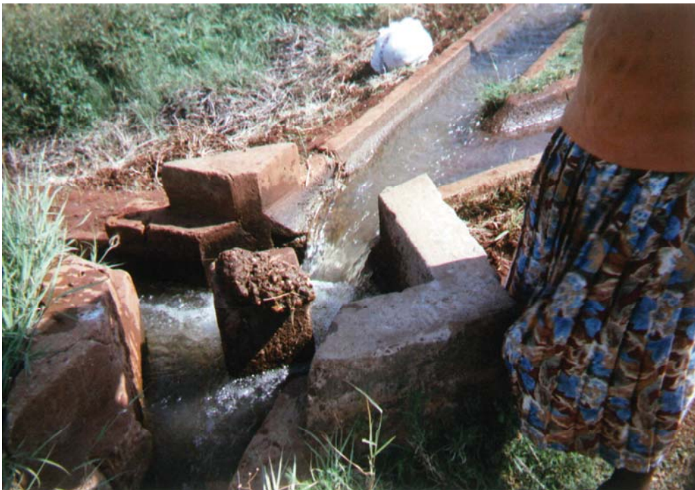
This is an intersection of secondary canals in bloc 3. (Participant de Nzhelele n°51, Mphephu, 2008)
