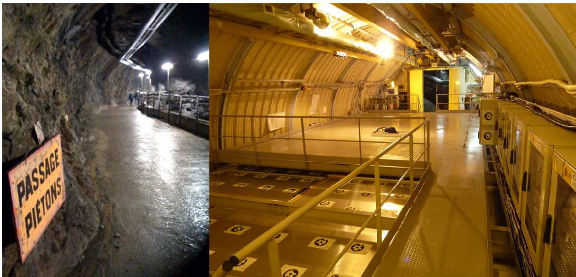
Figure 3.2: Picture of the tunnel underneath the hill (left) leading to the Double Chooz far laboratory (right). The installation was almost completed when the picture was taken.
