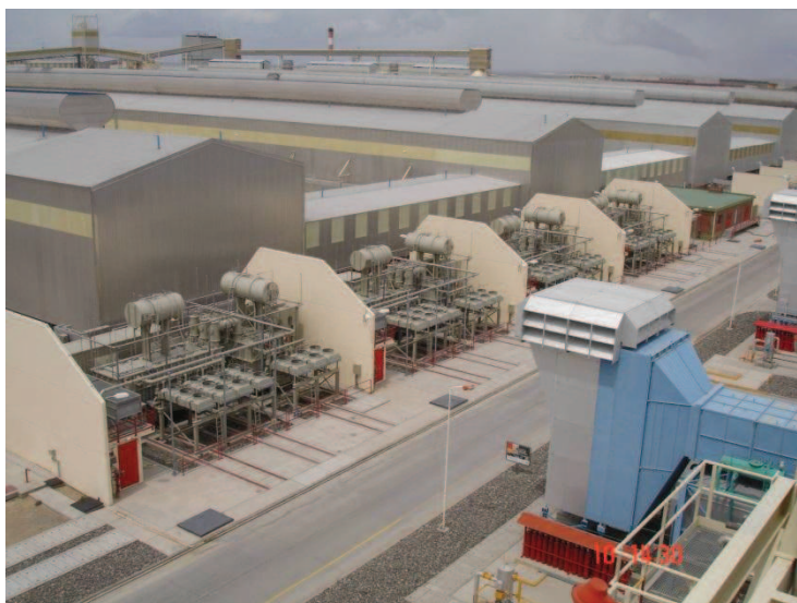
Figure 21. Example of an Alstom Grid AC/DC conversion substation (Aluar, Argentina)
