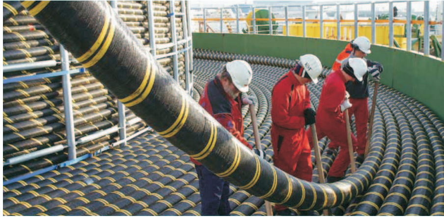
Figure 1.7: Underwater power transmission cables. Source: [15].
