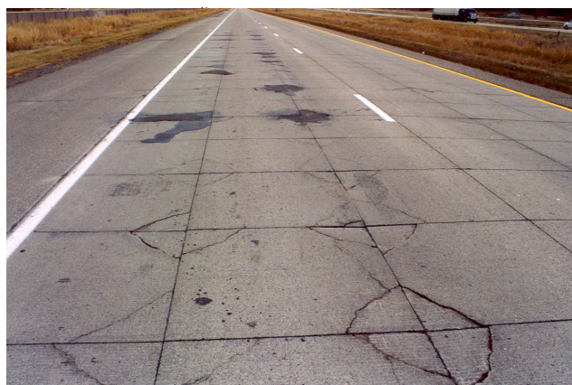
FIGURE 2 – Fissure au coin de dalle BCCM - Minnesota, USA [Burnham, 2005]
