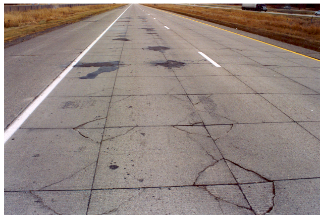
FIGURE 1.22 – Fissure au coin de dalle [Burnham, 2005]
