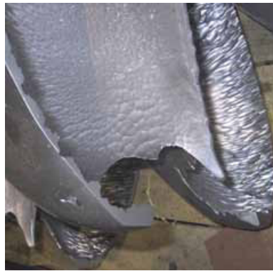
Figure 5.16. Damages on Pelton runner, Malana, India (credit: ANDRITZ HYDRO).
