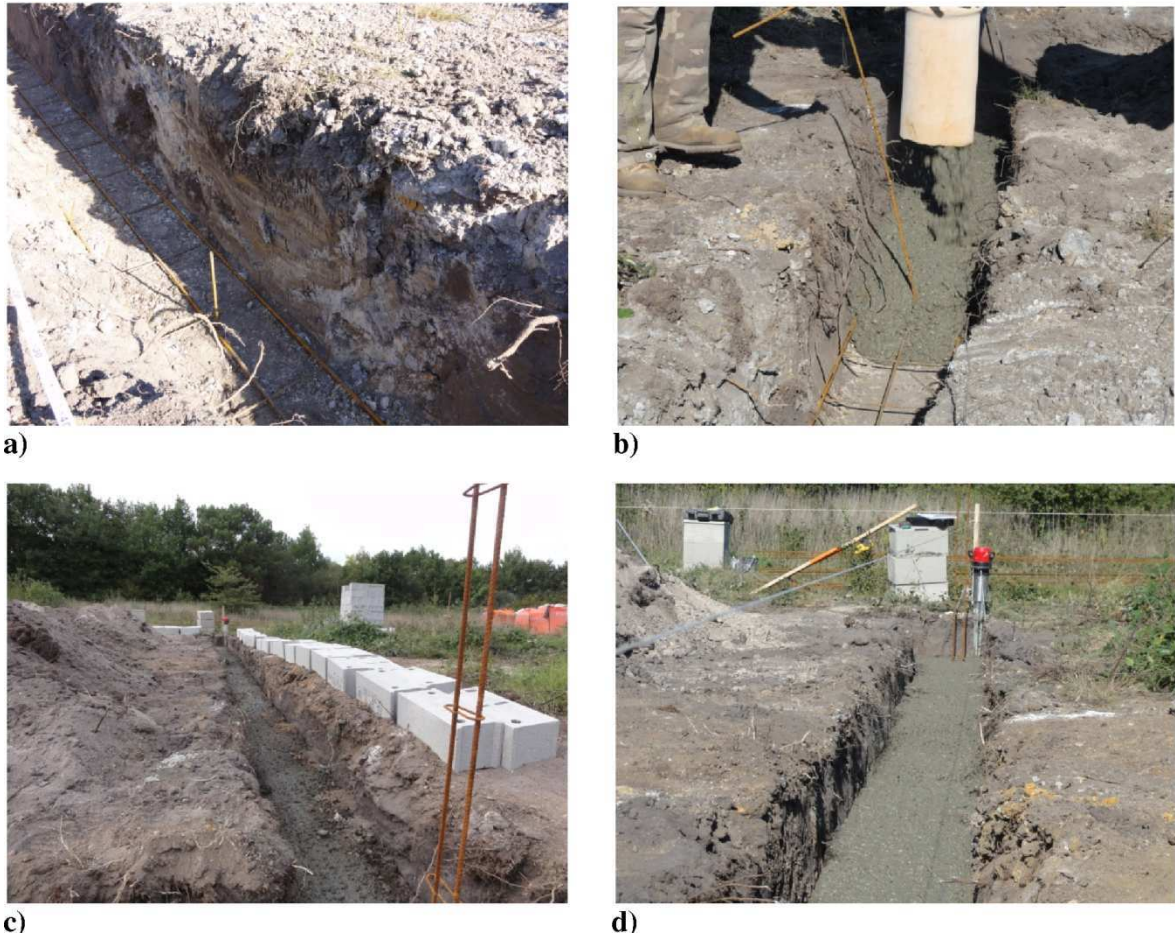
Figure 2-2: Different construction stages of the spread footings on the experimental site of Pessac
