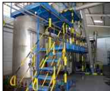
Photo 143 – Atelier de distillation
