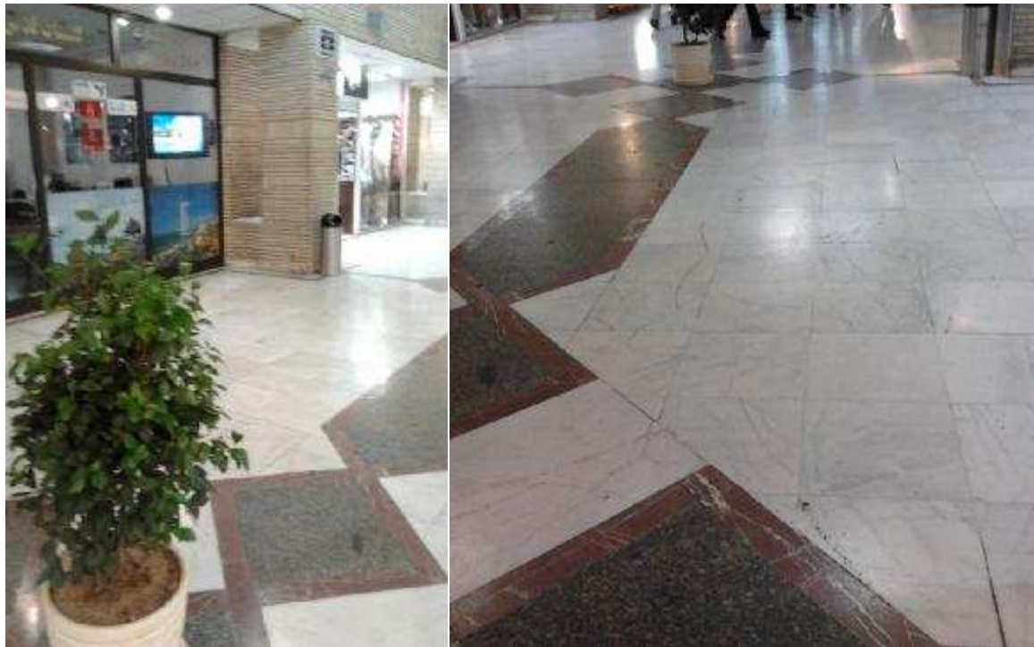
The surface in Golestan shopping center is white ceramic tile in a simple combination with colored tiles
