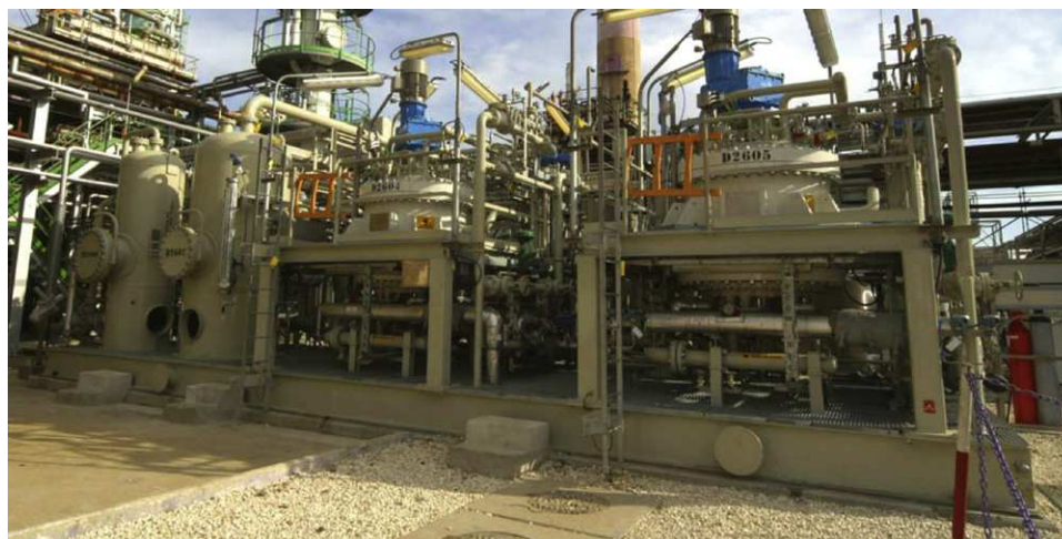
Fig. 7. Refinery application of RCPSA™ technology (courtesy of Xebec, www.xebecinc.com ).
