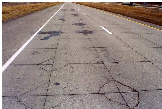
FIGURE 1.22 – Fissure au coin de dalle [Burnham, 2005]
