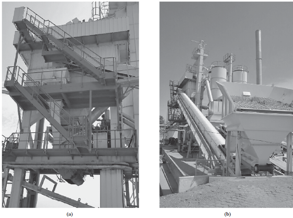
FIGURE 6 Industrial asphalt plant dedicated to LEA mixture in France.
