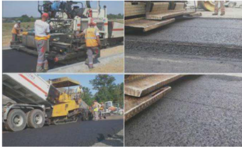
Figure 16. Paving GB50/14 mm with Noubleau aggregates and 35/45B bitumen in the Tours area. In-place density: 96.4%; stiffness modulus measured in indirect tension configuration E^*(15^\circ\text{C}-10\text{ Hz}) : 14,100 MPa.
