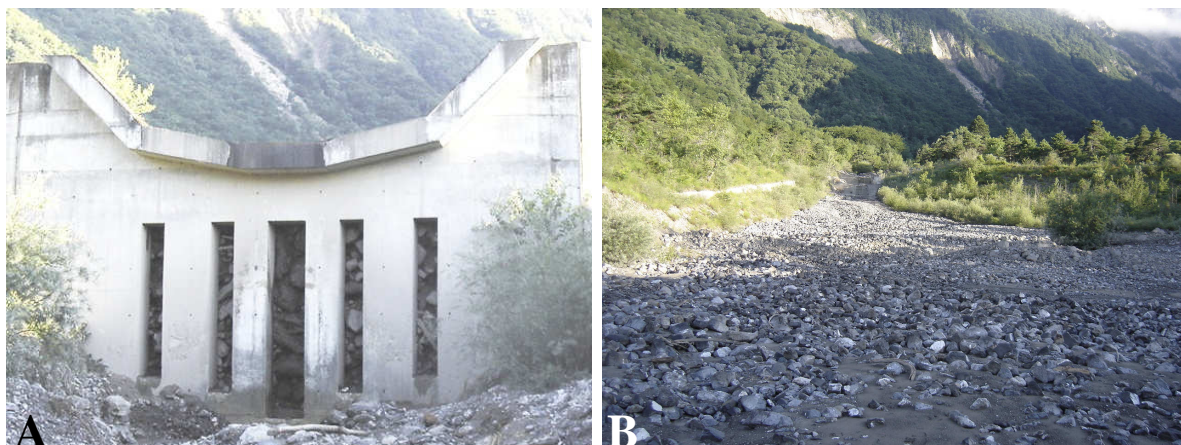
Figure 20 View of the sediment trap after a debris-flow with (A) the dam blocked by the boulder front with tree debris and (B) the rest of the trap filled with finer sediment.
