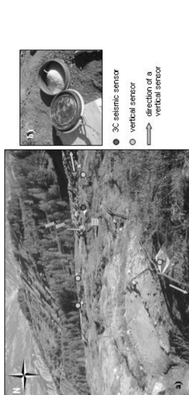
Fig. 1 – Seismic array permanent installation at Super-Sauze landslide: (a) array organisation and (b) detail of one box containing one sensor and filled with rice to prevent from humidity problems.
