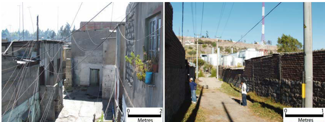
Figure 4.46: The majority of power is distributed overhead in Arequipa where lines are held up by reinforced concrete and wooden power poles.
