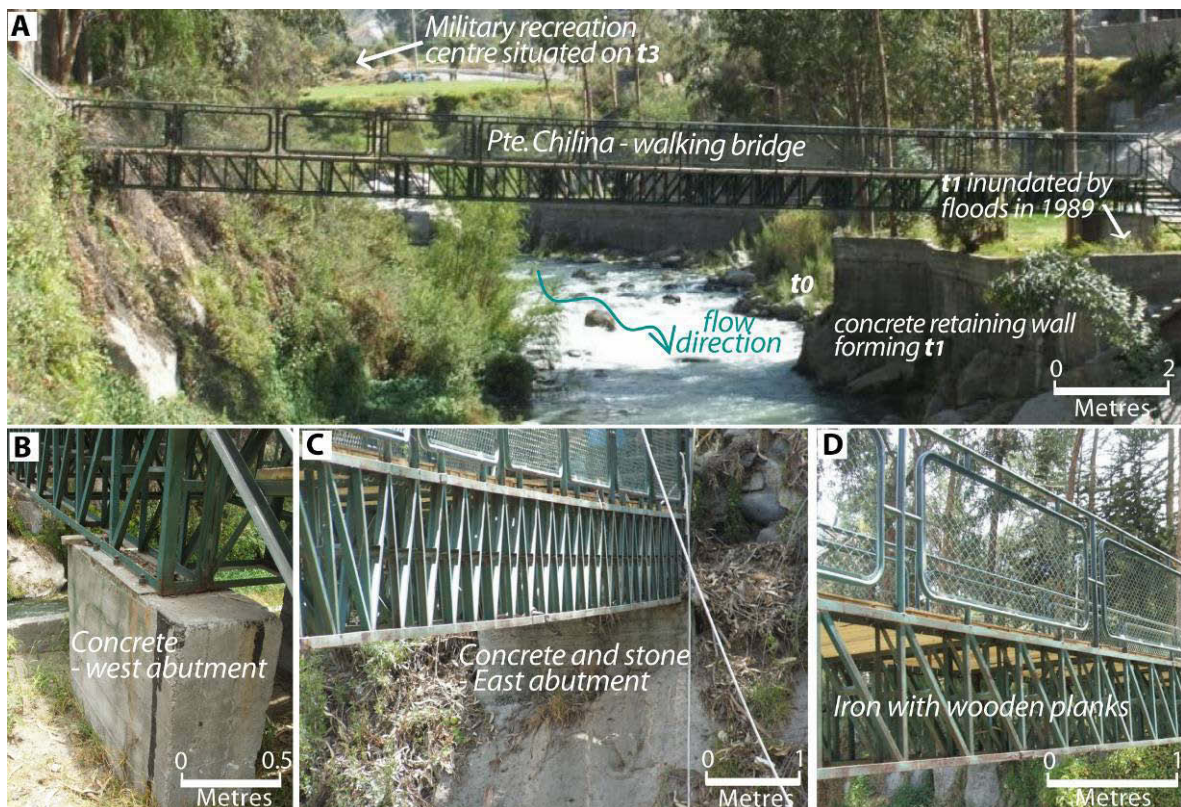
Figure 4.38: A: Looking upstream at the Chilina Walking Bridge. This bridge connects private land from one side of the river to the other. B: Reinforced cast in-situ concrete east abutment; the steel truss is bolted onto the concrete. C: Reinforced cast in-situ concrete west abutment built flush into the river bank. D: The steel frame truss with wooden plank bridge span.
