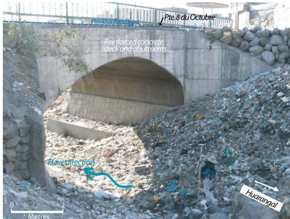
Figure 4.44: Upstream of Pte. 8 du Octubre in Huarangal. Of note is the amount of debris (including sediment, rock, building materials, rubbish) present in the channel. The GPS antenna is 2 m in height.
