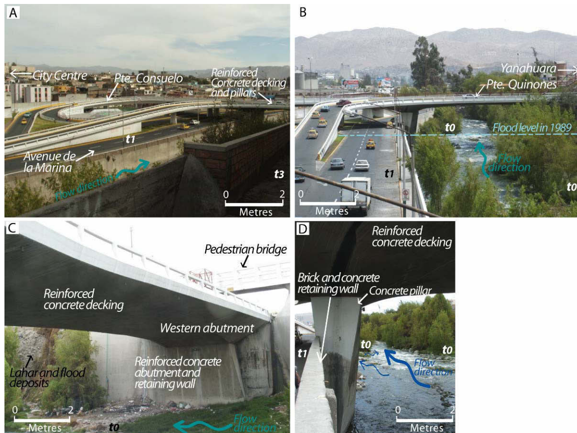
Figure 4.43: A: Looking downstream to Pte. Quiñones and Pte Consuelo. B: Looking downstream at Pte. Quiñones. C: The western abutment of Pte. Quiñones. D: The middle pier between the Río Chili and Avenida de la Marina on the eastern side of Río Chili
