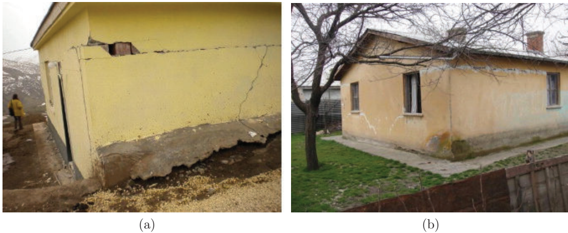
Figure 5.2: (a) Damage of a rural masonry building at Yukar Demirci Village, Turkey [16] (b) Failure of a rural masonry building in Palu, Turkey [16]
