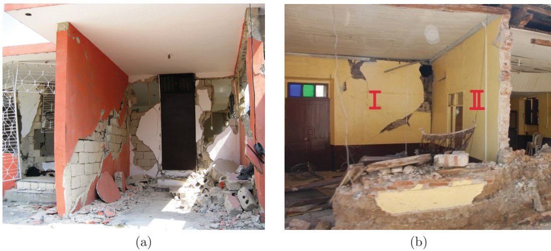
Figure 5.1: (a) Failure of masonry wall, Haiti earthquake (b) Out-of-plane collapse of masonry wall, Champerico, Guatemala
