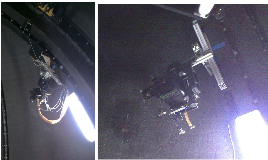
Figure 7.3: The pictures show the SkyDICE LED-head attached to the main arch of the SkyMapper dome at the end of its installation in June 2012.
