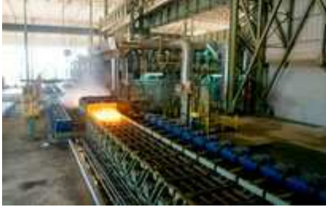
High pressure de-scaling box
