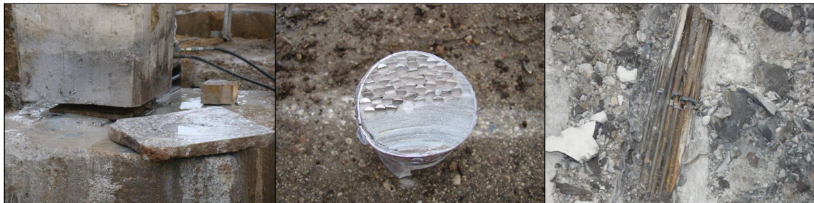
Figure 9.3 – Destructive damaging; a) cutting through one of the columns, b) and c) successive intersecting of prestressing tendons [VCE09].
