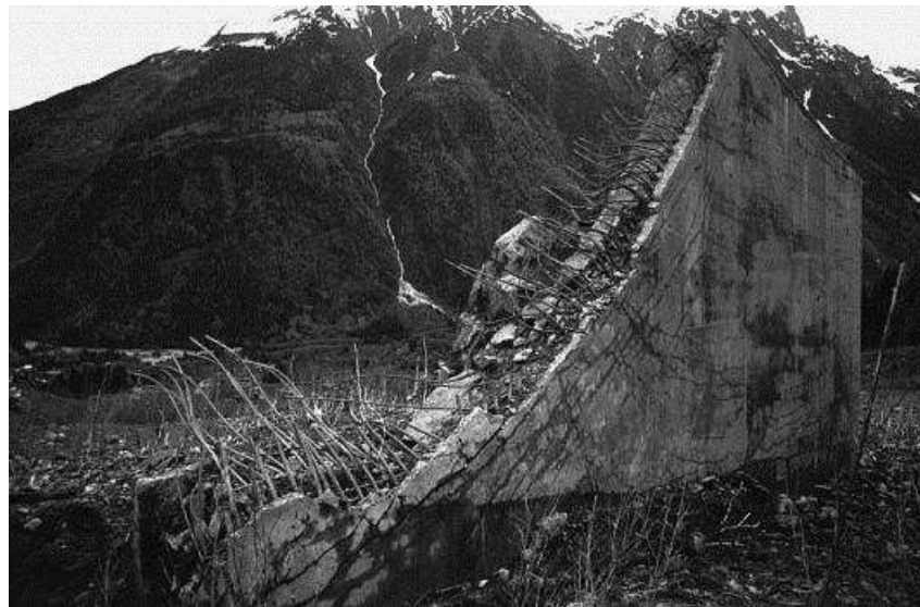
Figure 1: Deflecting wall in Taconnaz site destroyed by avalanche in February 11th, 1999 (image taken from Berthet-Rambaud et al. [4])
