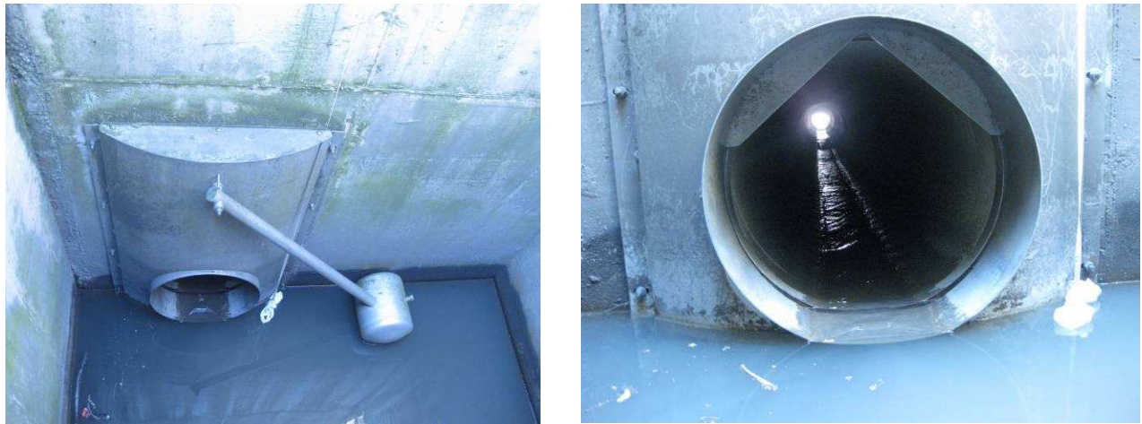
Figure 3-5 Outlet of Django Reinhardt detention basin equipped with regulator gate with a maximum outflow rate of 350 L/s (Hydroslide® gate)
