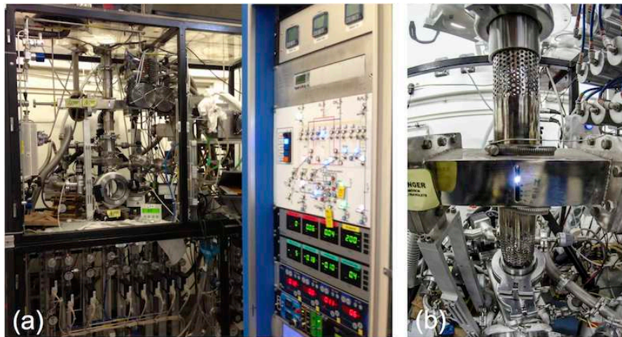
Figure 2.3: Pictures of (a) the whole MPCVD set-up with reaction and loading chamber on the left side and control panel on the right side and (b) the reaction chamber and microwave guide.
