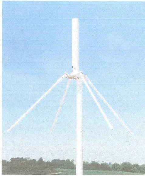
Figure 1.7: Ground-plane antenna used at the Champcueil station.
