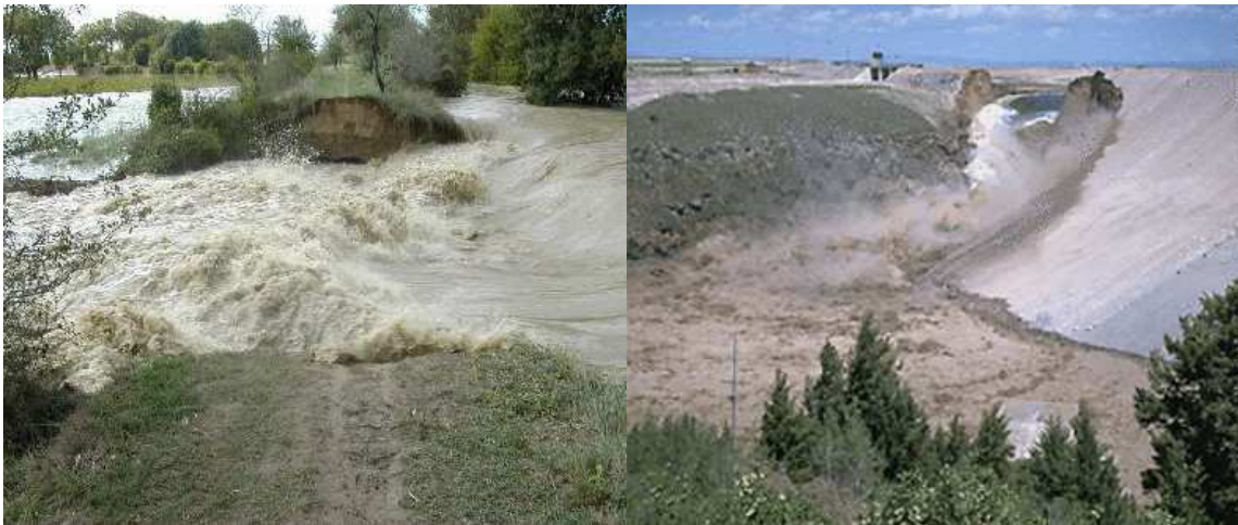
Figure 1.1. Breach caused by flooding of the Virdourle river in 2002 (left) and breach of the Teton Dam, 1976 (right).
