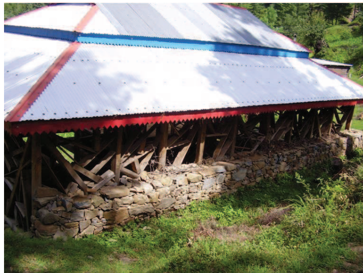
Figure 8.11 — The corners of this stacked stone wall have already started losing the stones.
