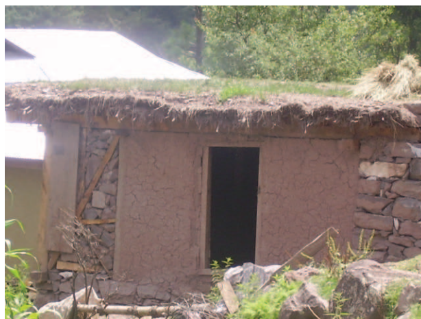
Figure 6.6 — A small room made in dhajji but with flat roof, used for storage now. Source : S. Abidi
