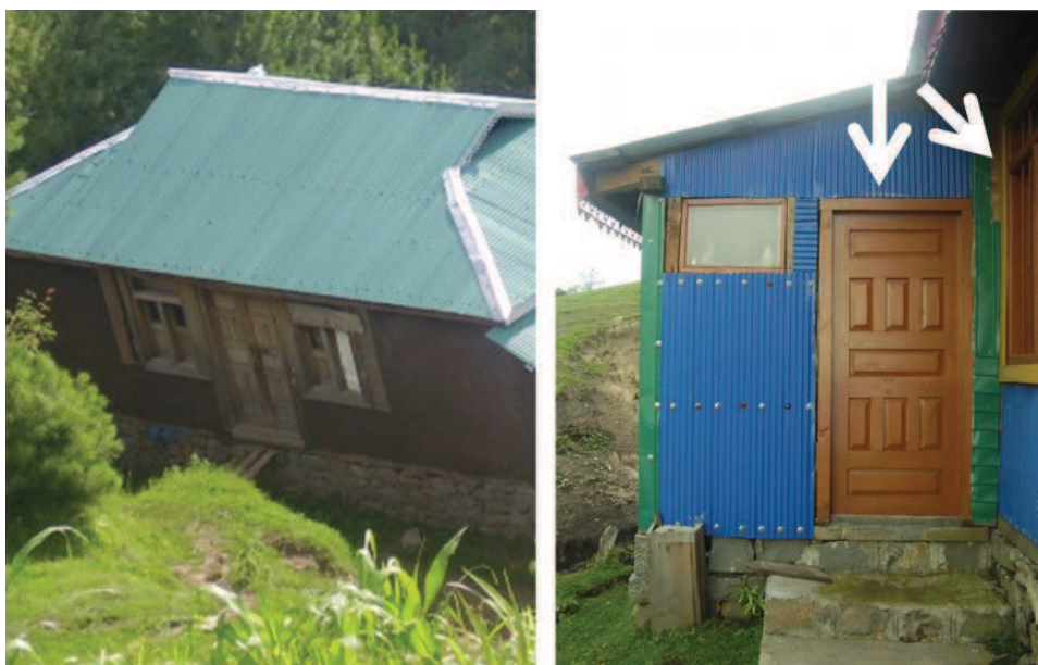
Figure 7.39 — Openings closer than 24 inches to each other or from the corner source : S. Abidi
