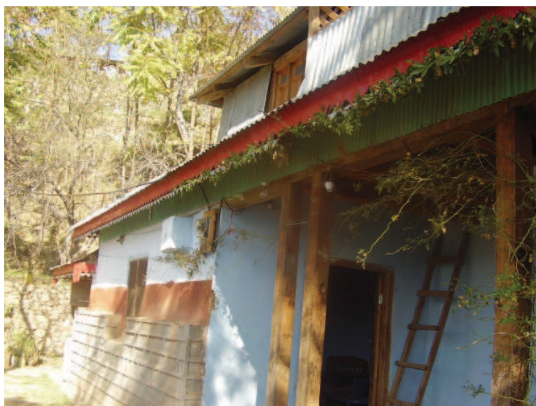
Figure 5.35 — Concrete blocks are not part of the structure. Source : S. Abidi.
