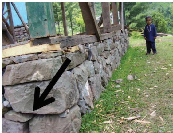
Figure 8.24 — Plinth issues. Source : S. Abidi
