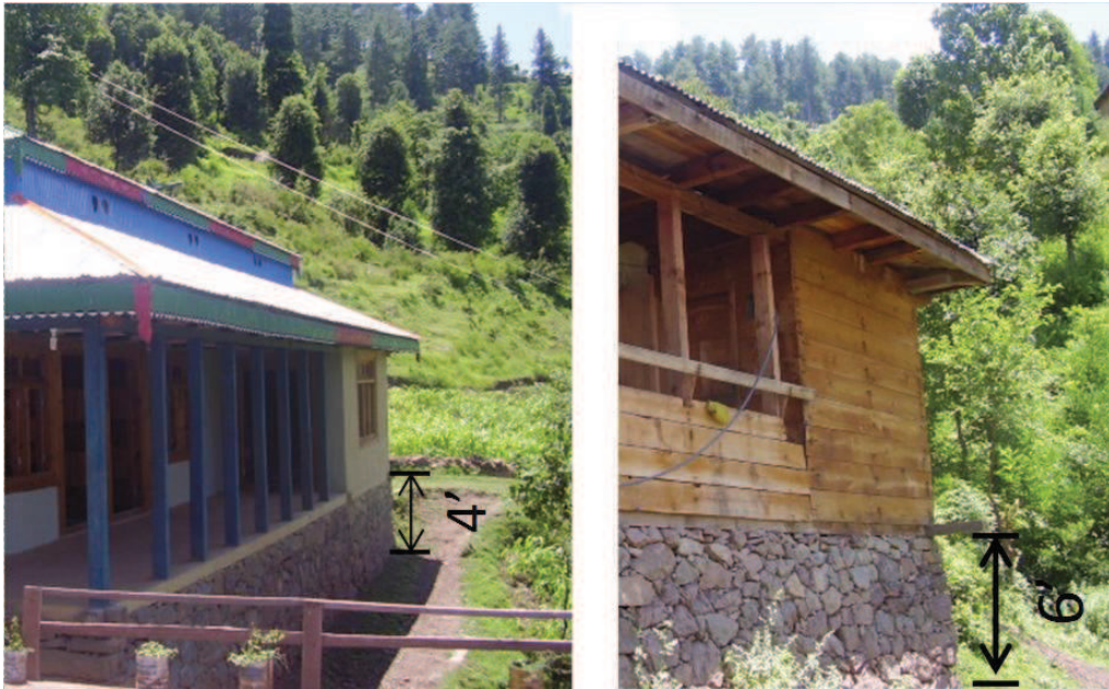
Figure 7.27 — more than 3 feet plinth height. Source : S. Abidi.
