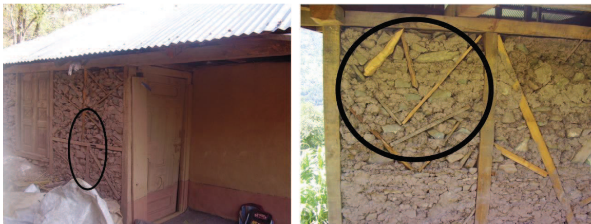
Figure 7.34 — Left : Discontinuous stud ; Right : No connection between bracings. Source : S. Abidi
