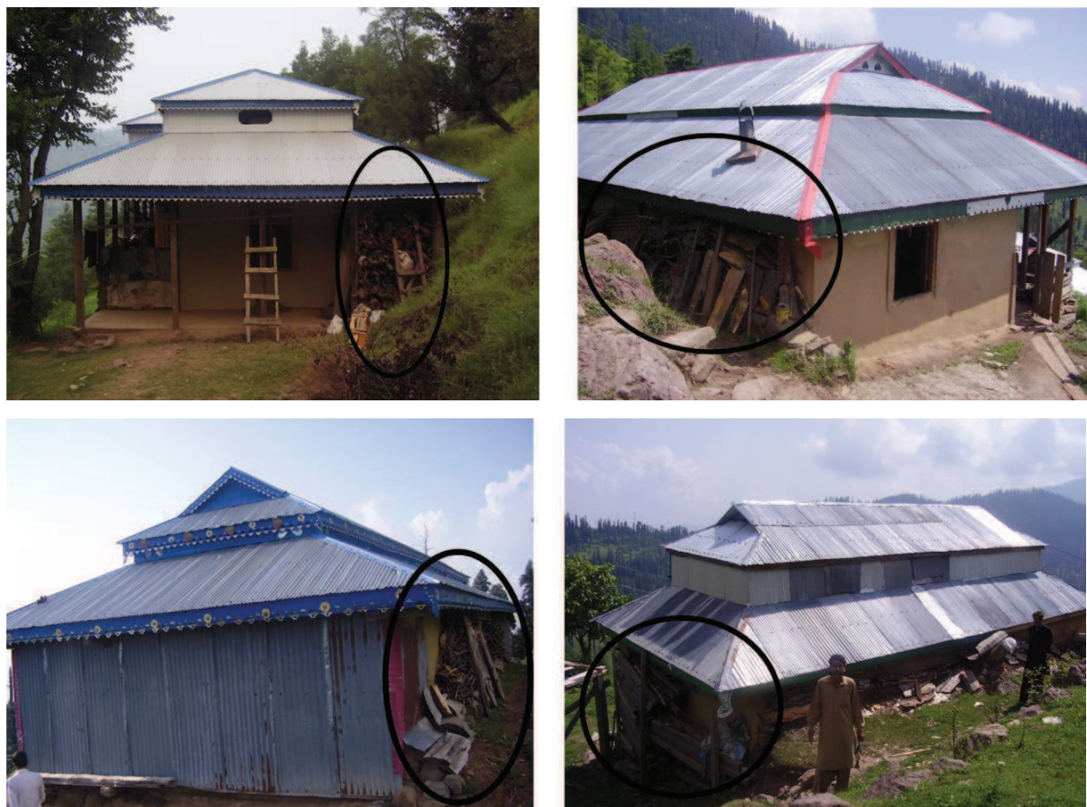
Figure 7.16 — Timber is stored beside the dhajji wall hence making the structure susceptible.
