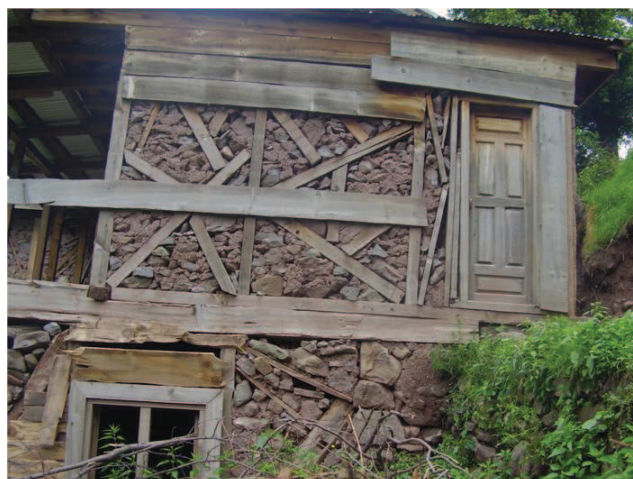
Figure 7.35 — Example of large distance between studs, under/over sized bracings and lack of connections. Although upper floor was treated with remedial measures, lower part has connection issues. Source : S. Abidi
