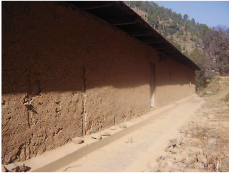
Figure 5.19 — Rear side of the market is having entrance door for school on first floor. Mud plaster is hiding the dhajji wall details however wooden posts (columns) are visible wherever the plaster is fallen. Source : S. Abidi
