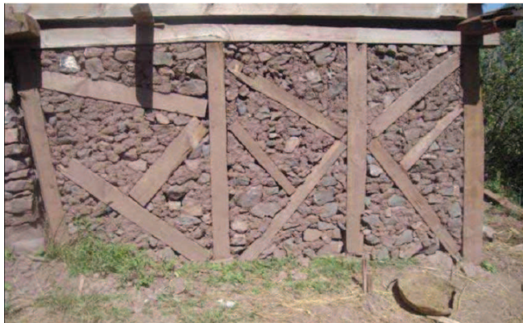
Figure 7.33 — Non compliant construction due to size of bracings, larger distance between studs and poor connections. Source : [Schacher, 2006]
