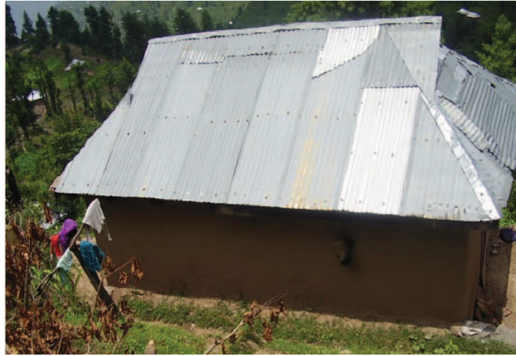
Figure 7.17 — Small pieces of CGI sheets are fixed through nails and bolts. Source : S. Abidi
