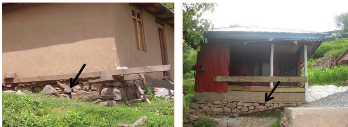
Figure 7.29 — During surveys, gaps were found in the plinth. Source : S. Abidi.
