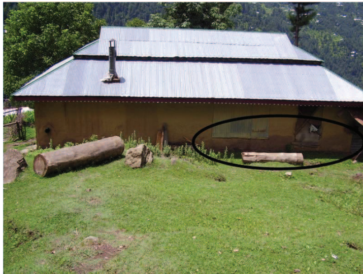
Figure 7.26 — Wall is Showing dampness which can be observed by its changed color. Source : S. Abidi
