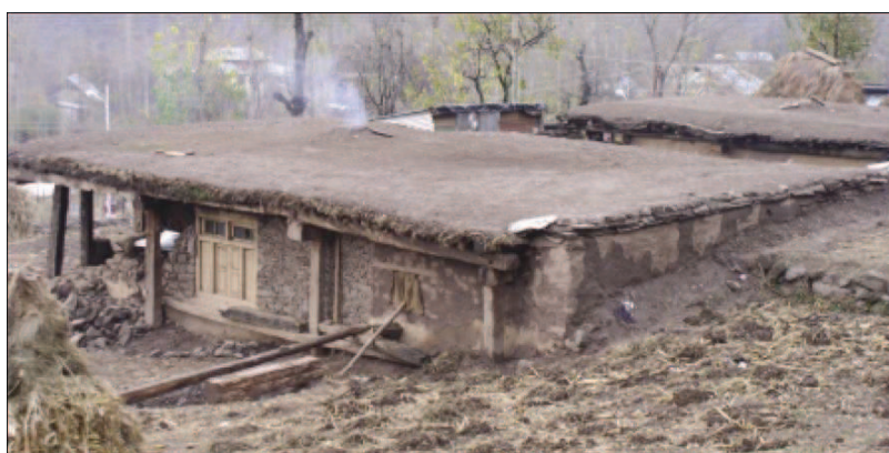
Figure 6.4 — Traditional flat mud roof on timber under structure with stone masonry walls.
