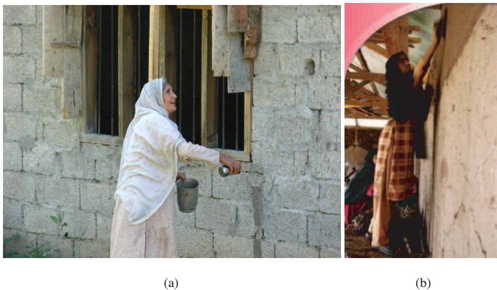
Figure 5.44 — Women also participated in reconstruction activities. (a) Source : ([Gallery, 2007]) ; (b) Source : ([UNHABITAT, 2007]) .
