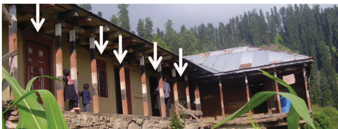
Figure 7.38 — Too many openings in the wall. Source : S. Abidi
