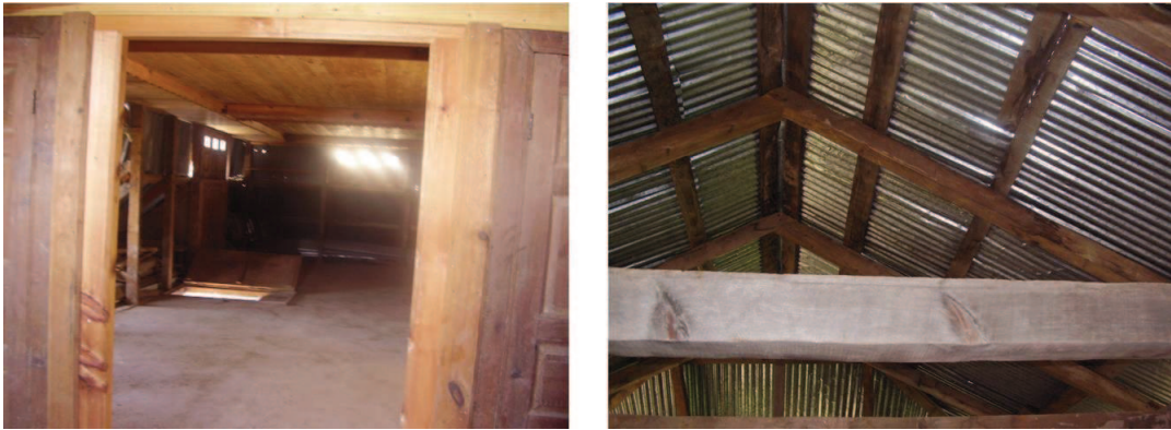
Figure 6.75 — Left : A ceiling is added to make a user friendly cuboid ; right : attic has a pitched roof. Source : S. Abidi.
