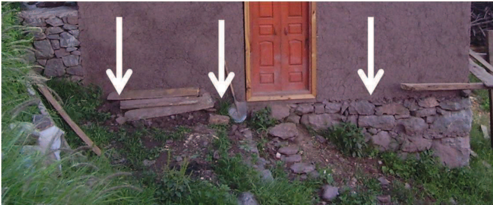
Figure 8.3 — Plinth issues. Source : S. Abidi
