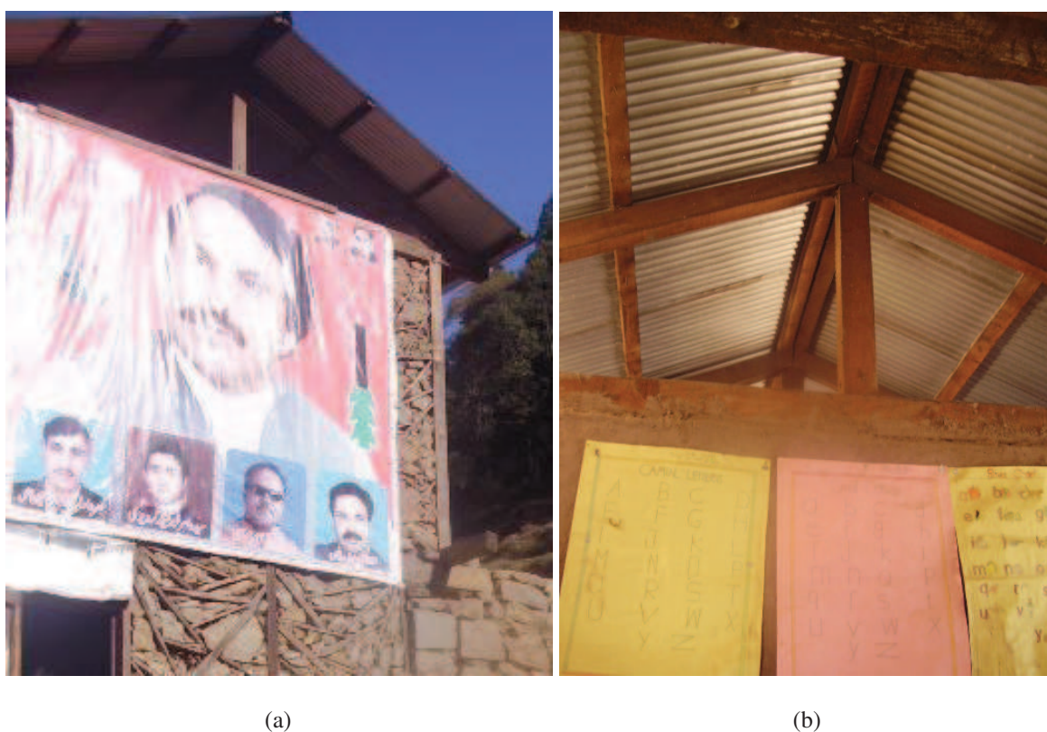
Figure 5.22 — Outside and inside views of the roof. it is not only open to the outside ; also it decreases the inner temperature because of its height. Source : S. Abidi
