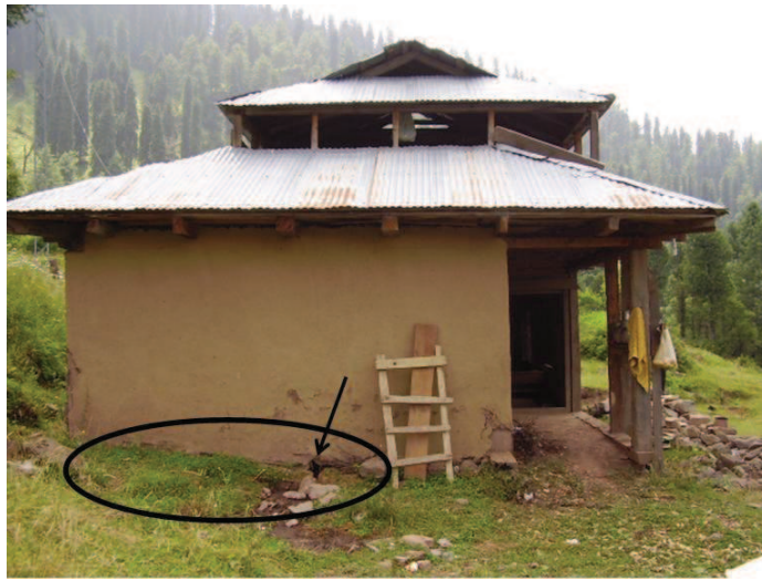
Figure 7.25 — Direct contact of walls with the ground. a hole is observed in the wall due to water seepage. Source : S. Abidi
