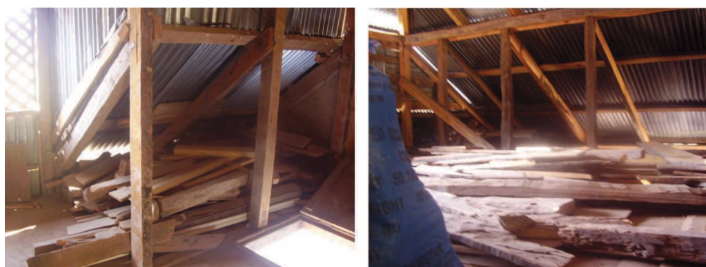
Figure 6.63 — Left : wooden logs and boards are stored in the eaves ; Right : planks are scattered on the floor. Source : S. Abidi
