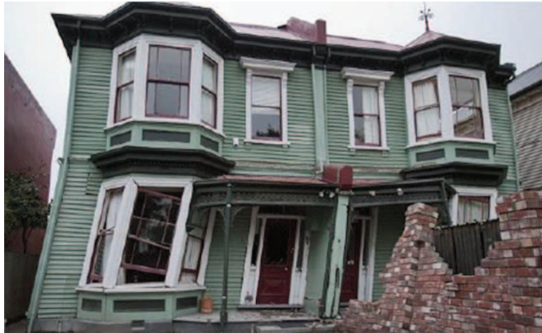
Figure 8.27 — A soft storey failure of a timber framed house not resulting in collapse. Source : [Morris et al. ]
