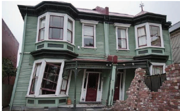
Figure 8.27 — A soft storey failure of a timber framed house not resulting in collapse. Source : [Morris et al. ]
