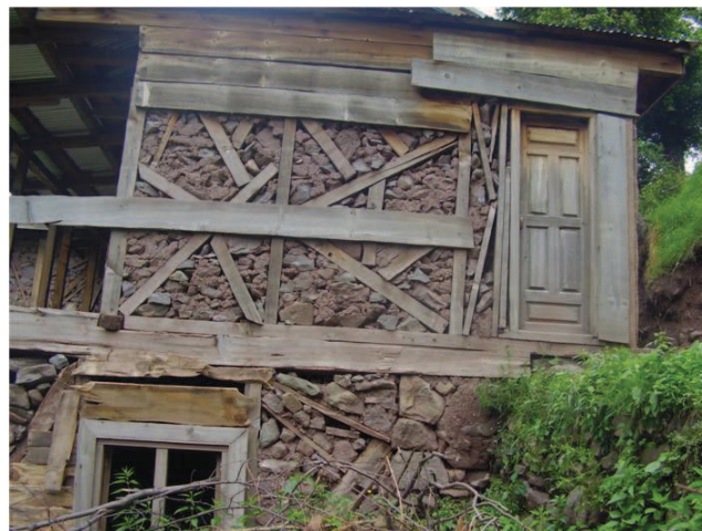
Figure 7.35 — Example of large distance between studs, under/over sized bracings and lack of connections. Although upper floor was treated with remedial measures, lower part has connection issues. Source : S. Abidi
