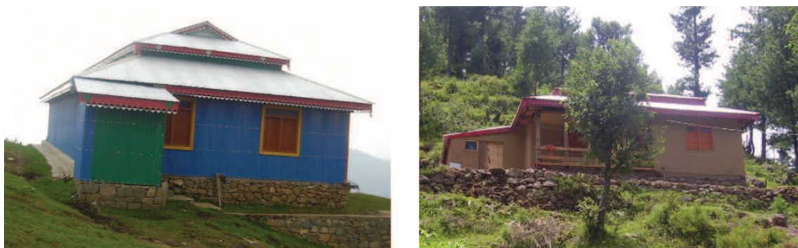
Figure 7.14 — Attached toilets and bathrooms belonging to higher income families. Source : S. Abidi
