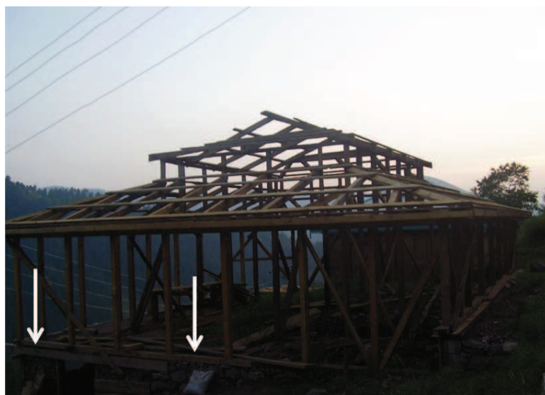
Figure 8.20 — Absence of retaining wall and presence of a dhajji built room beneath the house. Source : S. Abidi
