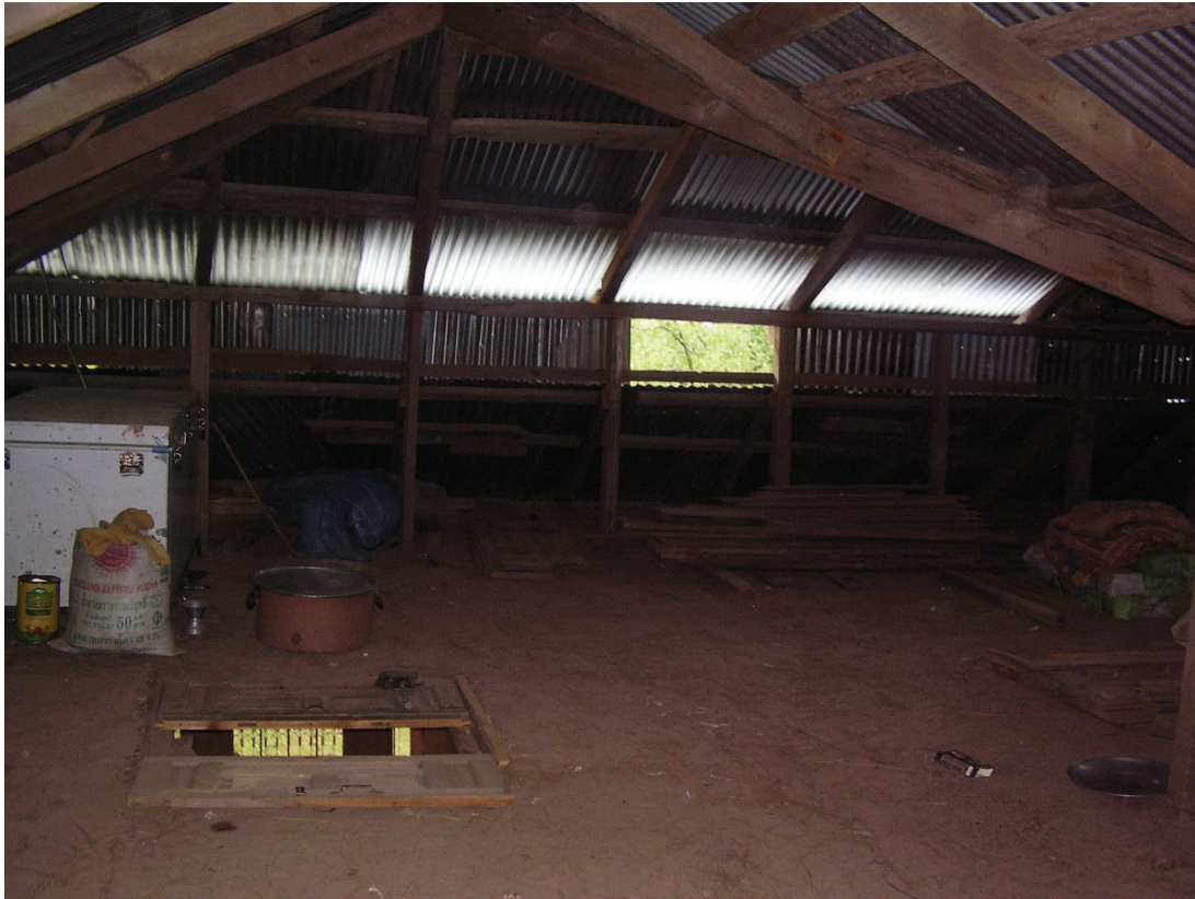
Figure 6.49 — A puncture in the floor of tower roof. Source : S. Abidi
