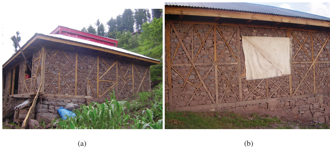
Figure 5.36 — The fabric in the right photo is hanging to cover open space for left window.
