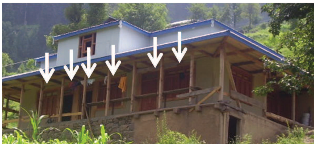
Figure 7.37 — Too many openings covering more than 50% of the wall area. All the openings are too close to each other. Source : S. Abidi
