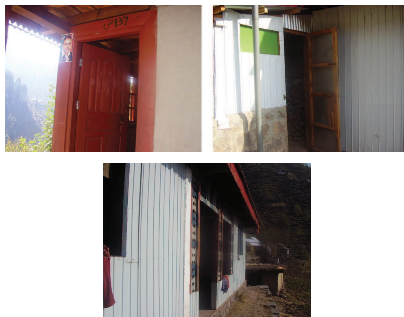
Figure 7.36 — : Vulnerability is increased due to too many openings. Source : S. Abidi
