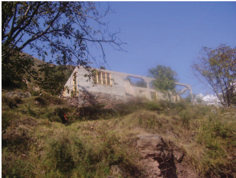
Figure 5.47 — An example of incomplete block masonry house in Kaimanja. Source : S. Abidi
