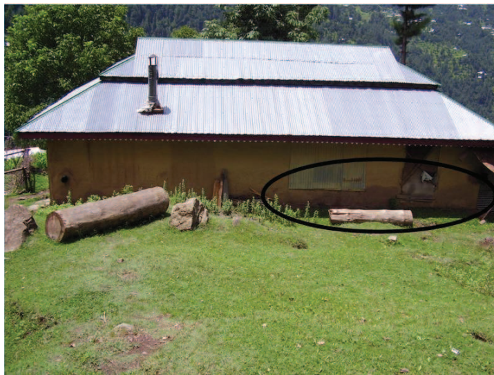
Figure 7.26 — Wall is Showing dampness which can be observed by its changed color. Source : S. Abidi
