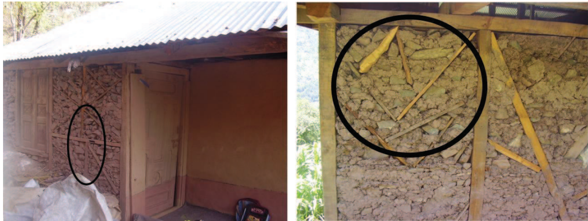
Figure 7.34 — Left : Discontinuous stud ; Right : No connection between bracings. Source : S. Abidi
