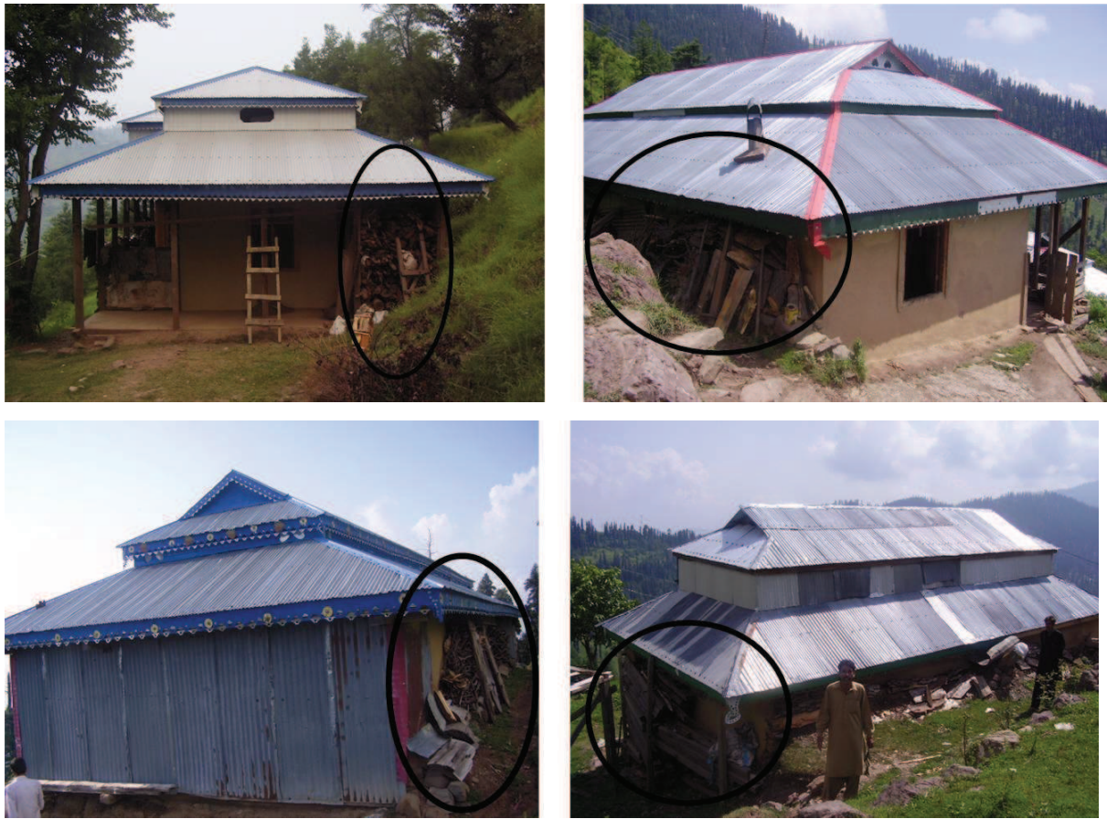
Figure 7.16 — Timber is stored beside the dhajji wall hence making the structure susceptible.
