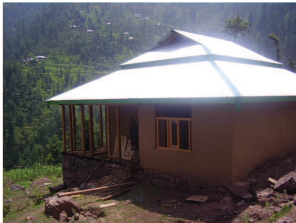
Figure 8.13 — Wall contacting ground directly. Source : S. Abidi
