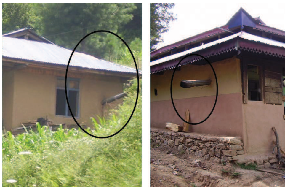
Figure 7.10 — Chimneys are hindering the outside passage. Source : S. Abidi
