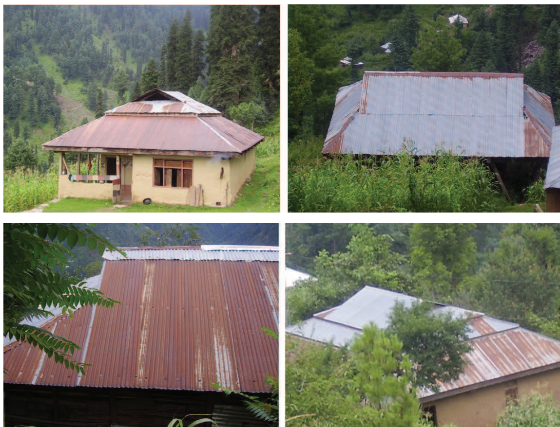
Figure 7.19 — The reconstructed houses are experiencing corrosion. Source : S. Abidi
