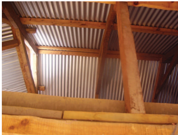
Figure 6.74 — A view of tower roof frame from the ground floor. no diagonal elements are observed. Source : S. Abidi
