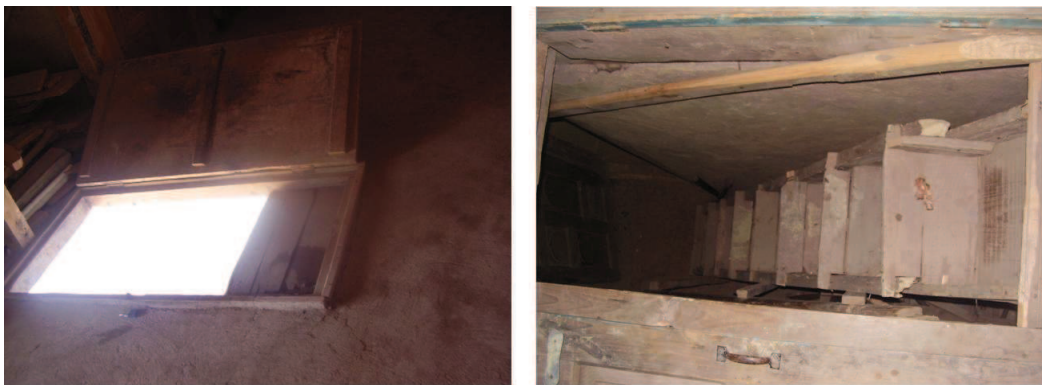
Figure 6.77 — The punctures in the ceiling to access tower roof. Source : S. Abidi
