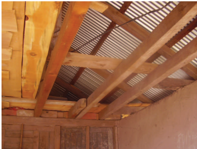
Figure 6.58 — User has to crawl in the attic where no reasonable height is provided. Source : S. Abidi
