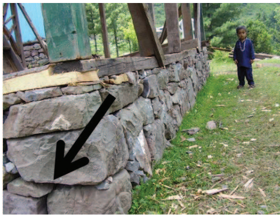
Figure 8.24 — Plinth issues. Source : S. Abidi
