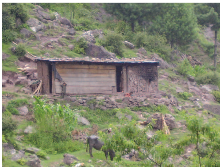
Figure 6.55 — Flat roof with no connections with the walls. Source : S. Abidi
