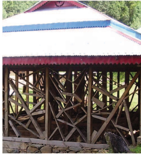
Figure 8.10 — Lack of proper connections between the bracing members. Source : S. Abidi
