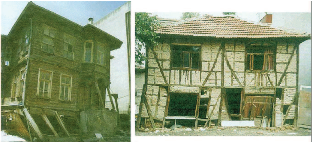
Figure 8.28 — Heavily damaged traditional wooden buildings due to soft story. Left : Large laterally displaced traditional building ([Bayulke, 2004]) ; Right : Laterally displaced traditional building ([et al, 1999])
