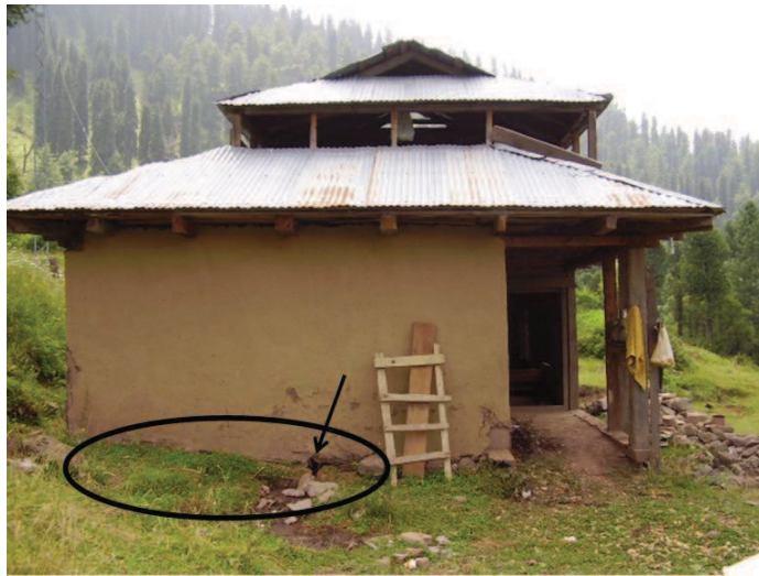
Figure 7.25 — Direct contact of walls with the ground. a hole is observed in the wall due to water seepage. Source : S. Abidi
