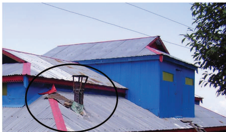
Figure 7.18 — As leakage from around the chimney was to be avoided, the owner has just put a small piece of CGI sheet and then put stone. Plastic is also surrounding the chimney. The owner was still facing water seepage. Source : S. Abidi
