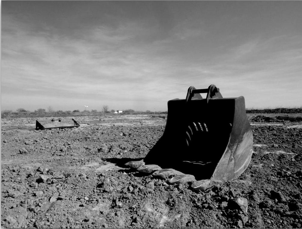
The Cassaïre site creation at large scale using a bulldozer to create topography.
