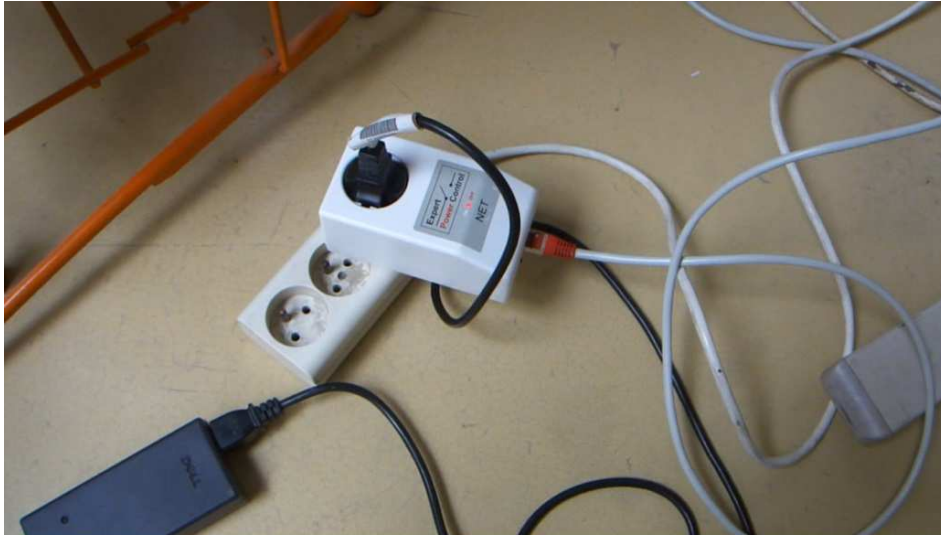
Figure 68 : prise programmable via port Ethernet
