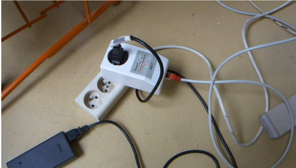
Figure 68 : prise programmable via port Ethernet
