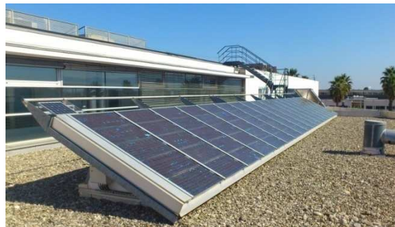
Figure II- 3: Installation photovoltaïque "Shed", PROMES-CNRS, Perpignan
