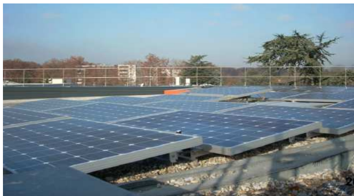
Figure II- 8: Toit "R+2" 29kWc, ADREAM
