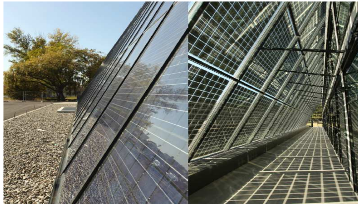
Figure II- 6: Façade photovoltaïque 36 kWc, ADREAM
